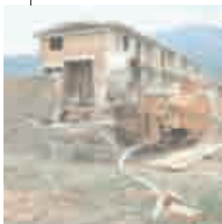
INDUSTRY AND BUILDING SITES Reliable power supply for machinery.
